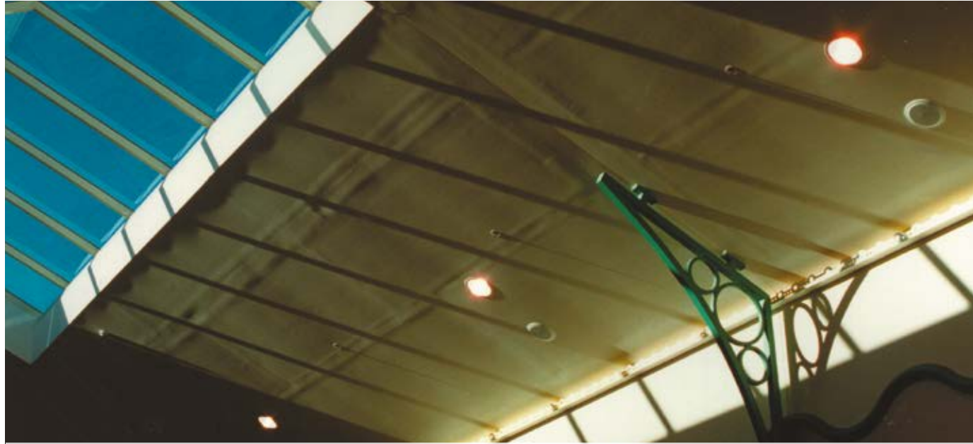
A plasterboard ceiling under glancing light conditions
