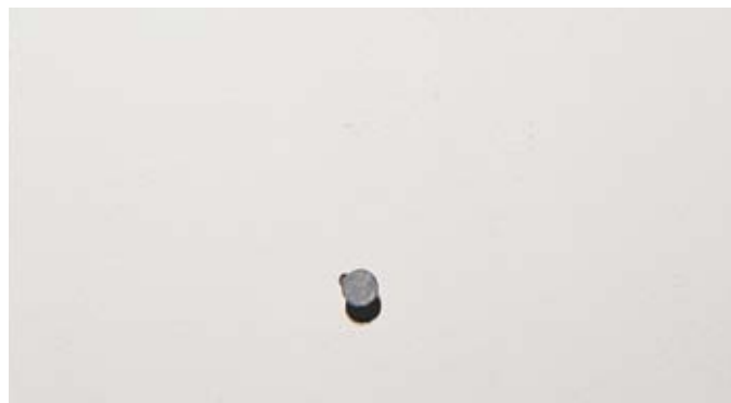
Plasterboard joint under diffused frontal light
